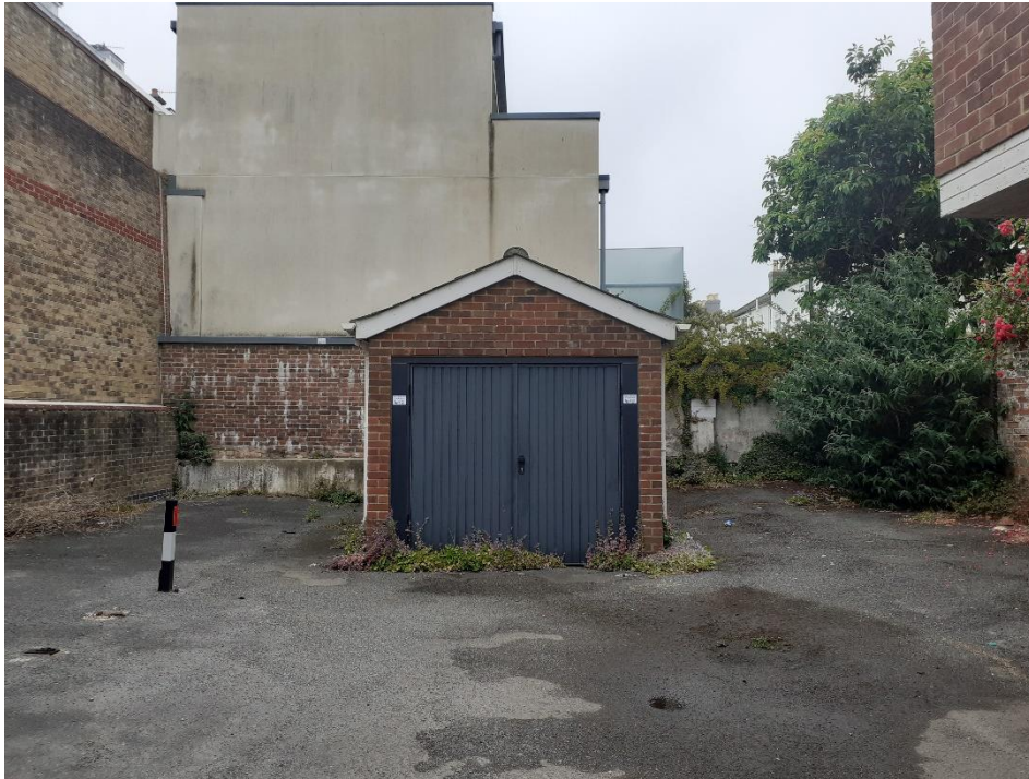
Existing Garage at northern end of rear car parking/garage area to the rear of 55-69 Centurion Road.
